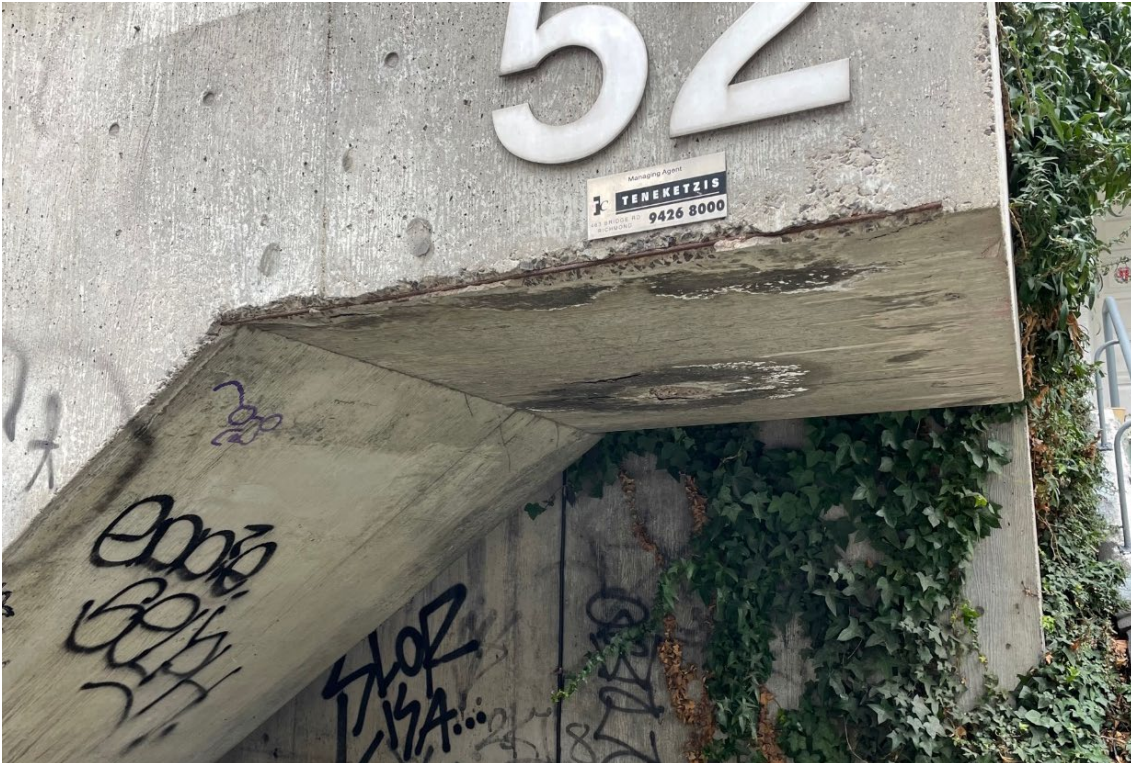
Figure 12 Localised failure of concrete finish
