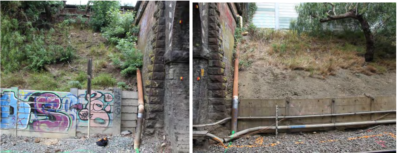
FIGURE 8: VIEWS OF LHS AND RHS APPROACHES AND THEIR INTERFACE WITH THE UP-END PORTAL. (SOURCE: ACG)
