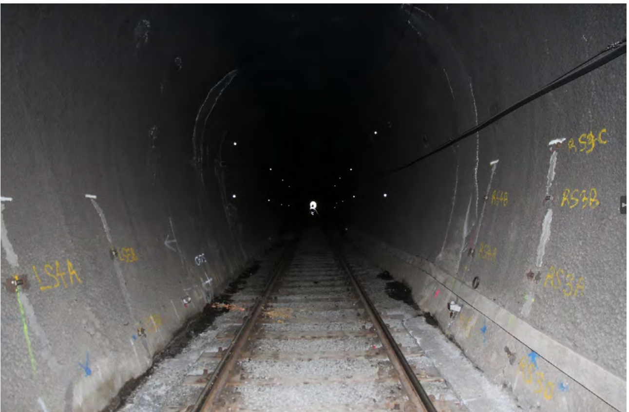
FIGURE 14: INTERNAL VIEW OF TUNNEL SHOWING CONDITION OF RELATIVELY RECENT SHOTCRETE – LOOKING SOUTH. (SOURCE: ACG) NOTE: TUNNEL STRUCTURAL DESIGN REPORT MENTIONED THIS SHOTCRETE ON WALLS AND PUMPING GROUT BEHIND LINING TO FILL VOIDS WAS DONE IN 1995.
