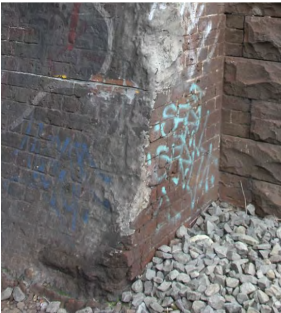
FIGURE 11 (LHS): VIEW OF DAMAGED BRICKS ON DOWN-END PORTAL. (SOURCE: ACG)
