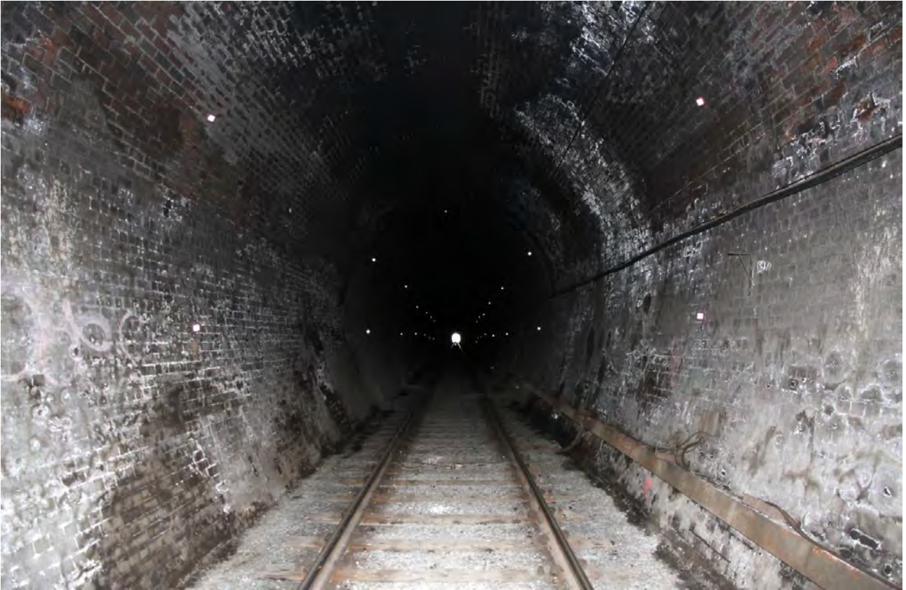
FIGURE 13: INTERNAL VIEW OF TUNNEL SHOWING CONDITION OF BRICK LINING, TRACK AND SERVICES – LOOKING SOUTH. (SOURCE: ACG)
