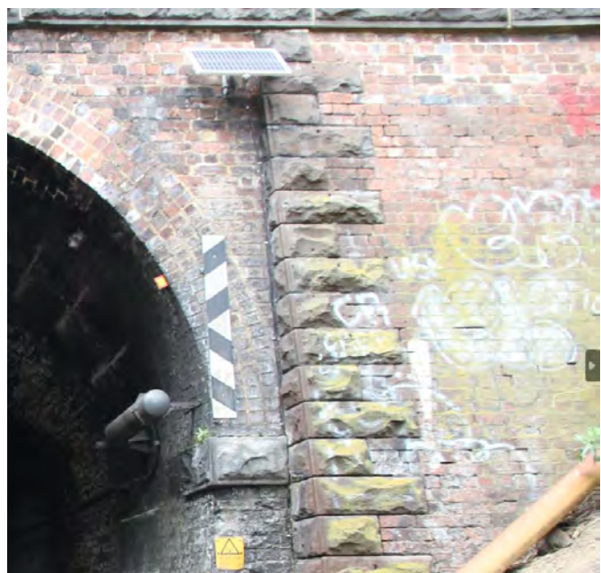
FIGURE 12 (RHS): VIEW OF UP-END PORTAL SHOWING DEGRADED MORTAR AND GRAFFITI. (SOURCE: ACG)
