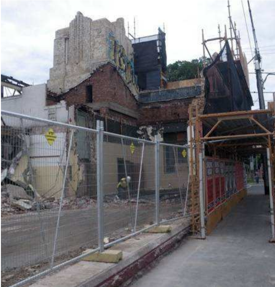
Figure 141: Victoria Parade and Brunswick St Cable Tram Engine House during demolition 2009. http://indolentdandy.net/fitzroyalty/2009/12/09/a-facade-of-heritage-values/
